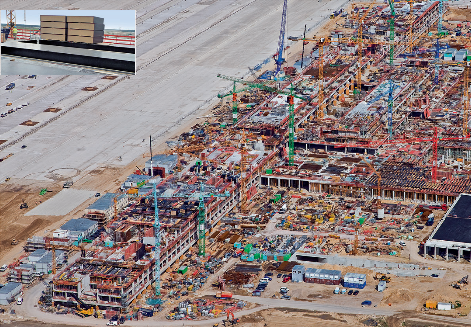
Customised slab tables for beams and box-outs for the construction of BBI Berlin Brandenburg International Airport, Berlin.
